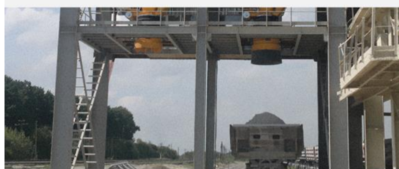
TRUCK/RAILCAR LOADING SPOUTS
